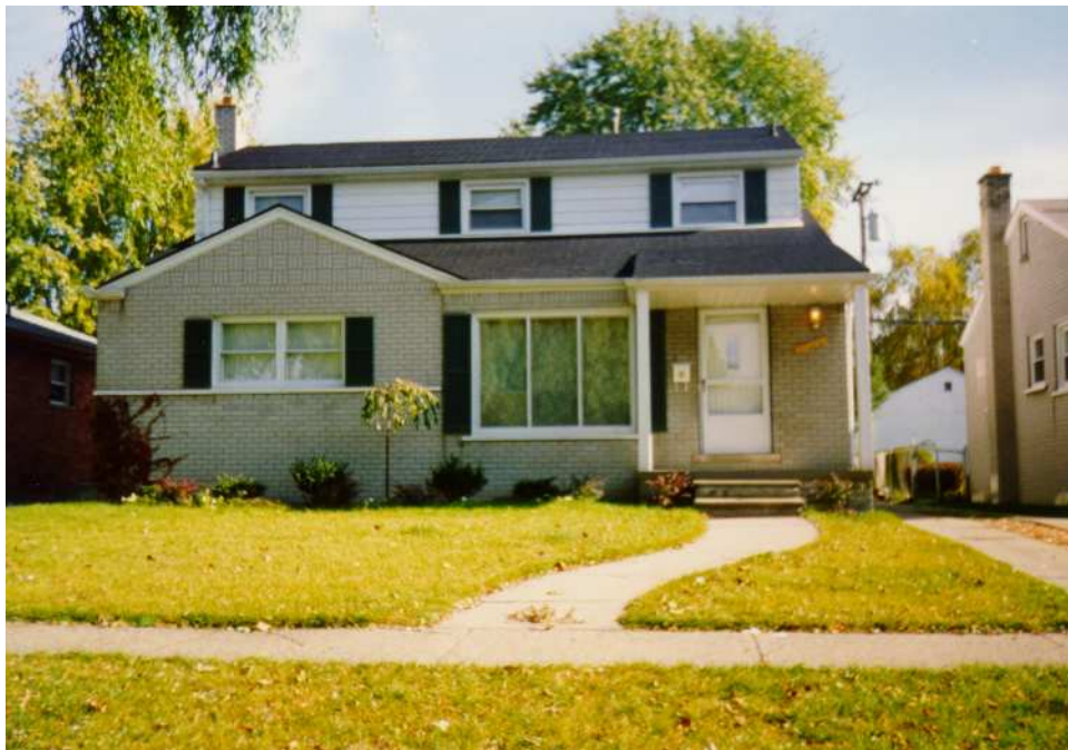
Standard ranch with the addition of a second story post-construction add-on. Could experience minor to major roof sag due to the addition, but not seen here.
