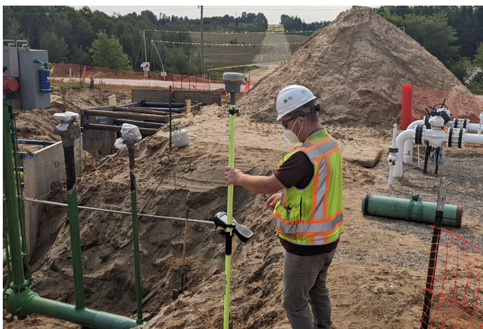
Figure 3. A precise GIS geodatabase of as-built pipeline data and orthometric aerial imagery of the pipeline corridor was created. Large datasets received daily data processing and network adjustments to achieve the centimeter-level accuracy and details required.
