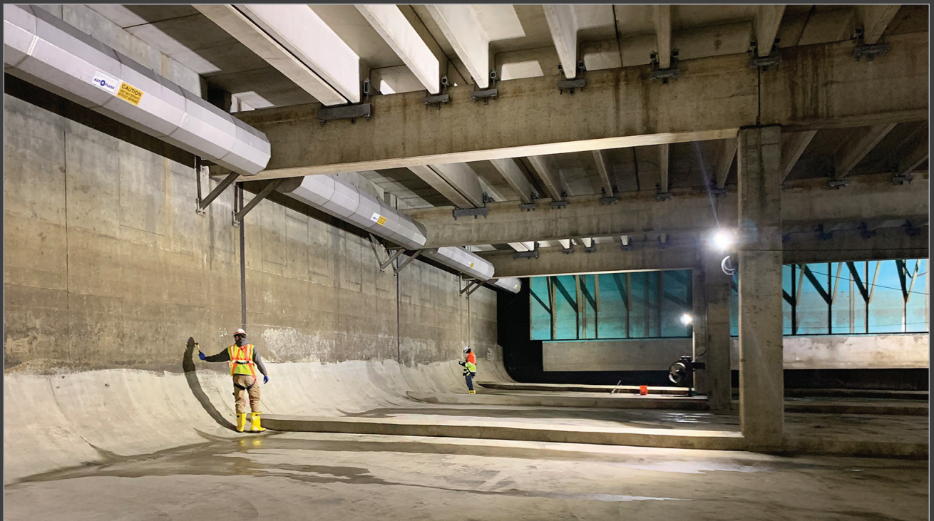
Leveraging a collaborative workflow, experienced structural engineers, and reality capture technology experts, the project team saved GLWA preparation time and cost that otherwise would have been necessary to assess the basins' concrete conditions. Photo courtesy of Wade Trim
