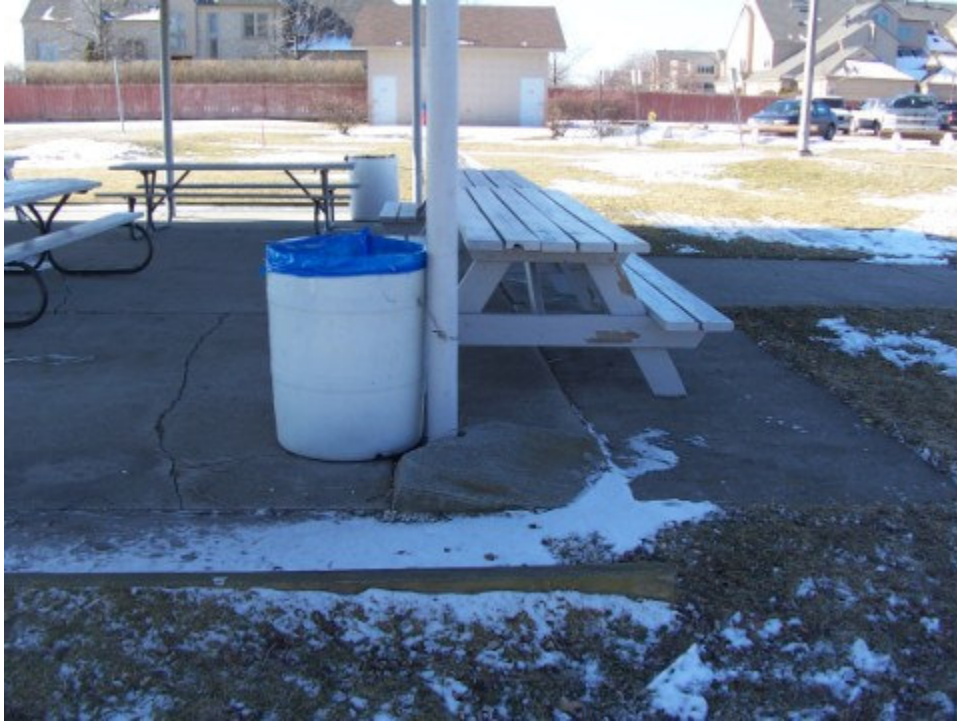
Photograph No. 11: Looking north at post #1. Note cracking and heaving of slab around pole.
