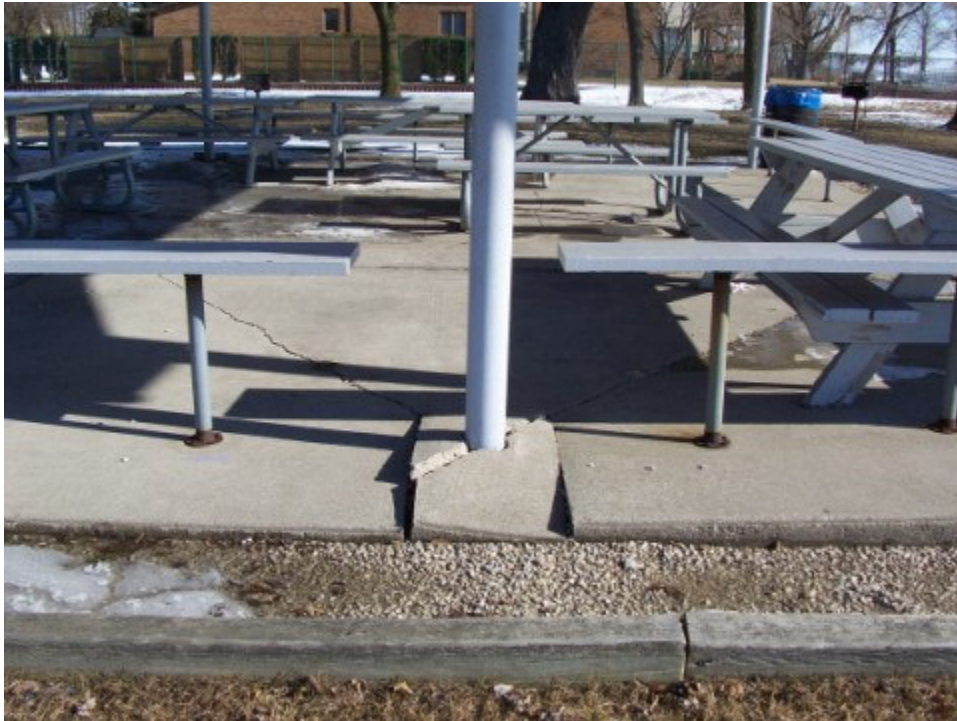
Photograph No. 2: Looking north at post #7. Notice heaving and cracking of slab around the pole.
