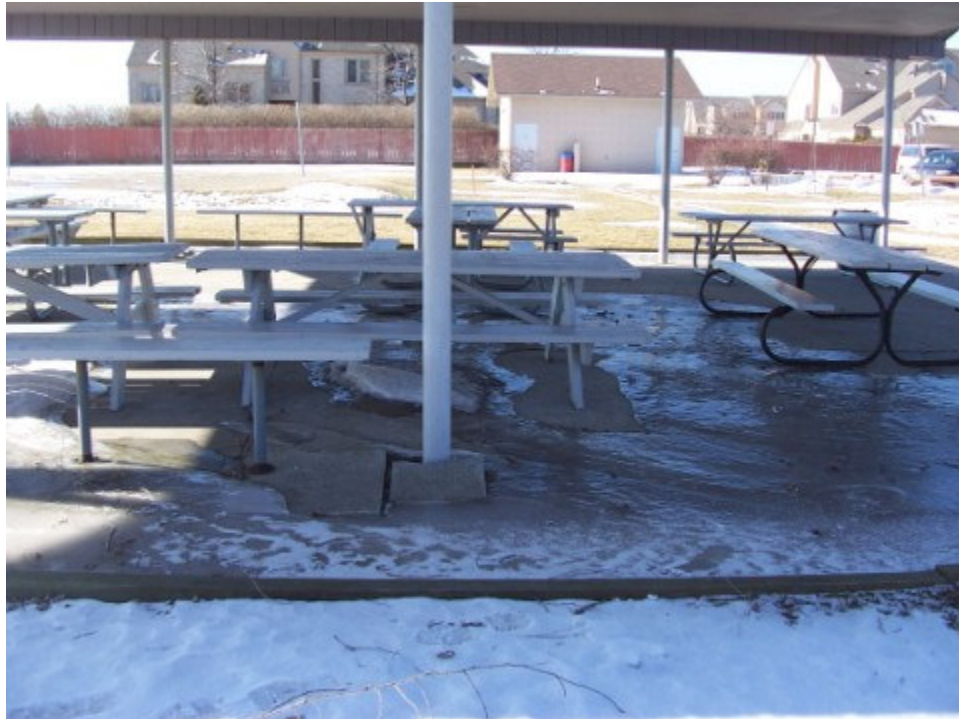
Photograph No. 9: Looking south at post #3. Note standing water and ice around perimeter of slab and across slab and cracking and heaving of slab around pole.
