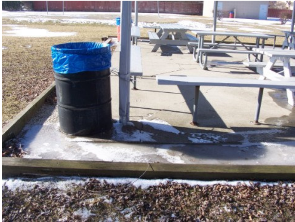
Photograph No. 7: Looking south at post #5. Note standing water and ice around perimeter of slab.
