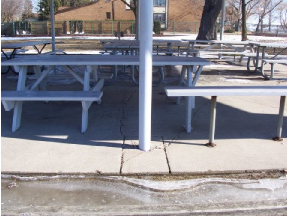
Photograph No. 5: Looking north at post #8. Note standing water around perimeter of slab, cracking of slab around pole, and cracking of slab within shelter footprint.
