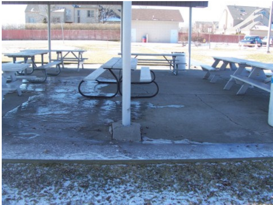
Photograph No. 10: Looking south at post #2. Note standing water and ice around perimeter of slab and across the slab and cracking of slab around pole.
