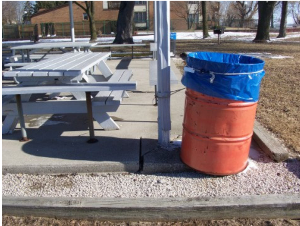
Photograph No. 3: Looking north at post #6. Note settlement and cracking of slab around the pole.
