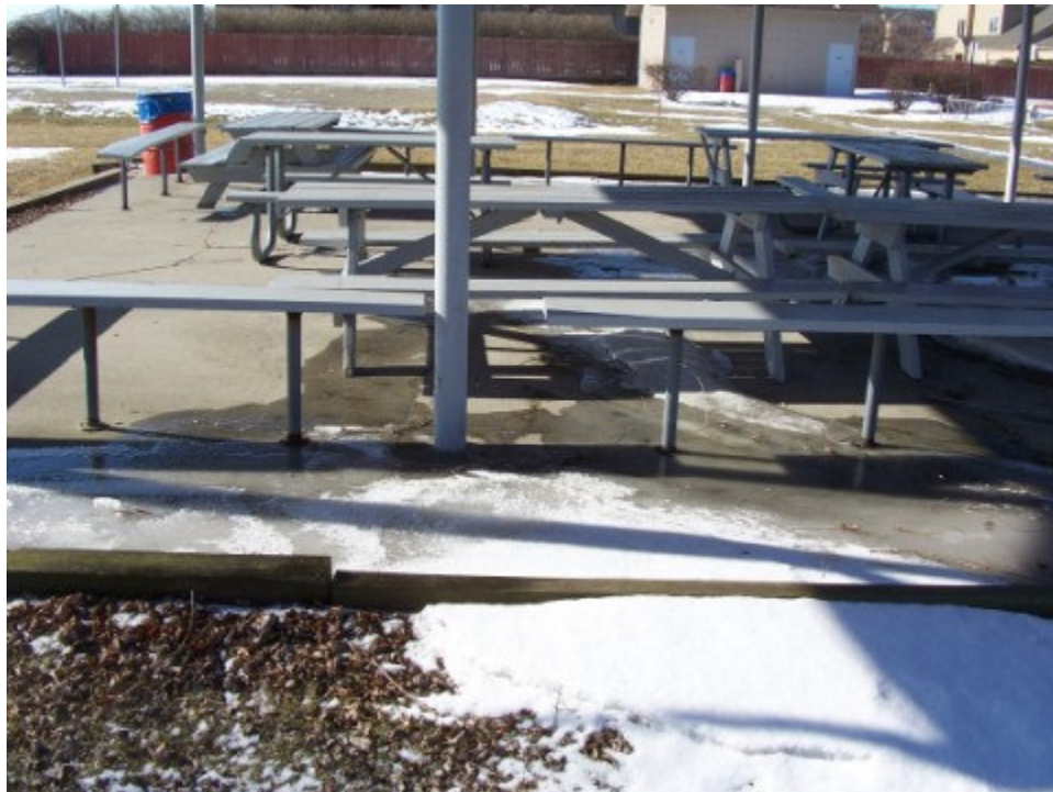
Photograph No. 8: Looking south at post #4. Note standing water and ice around perimeter of slab as well across the overall slab.
