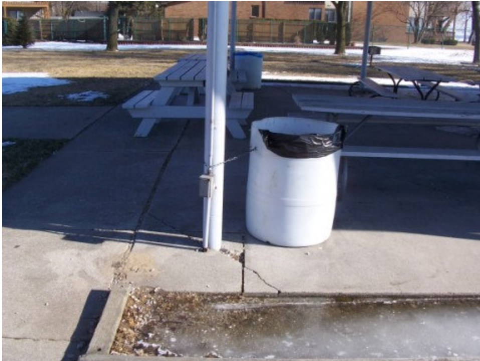
Photograph No. 6: Looking north at post #10. Note standing water around perimeter of slab and cracking of slab around pole.
