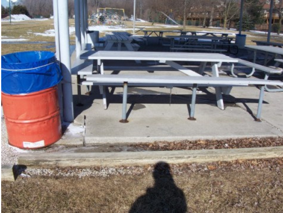
Photograph No. 15: Looking west at post #6. Note standing water and ice around perimeter of slab and cracking of slab around pole.
