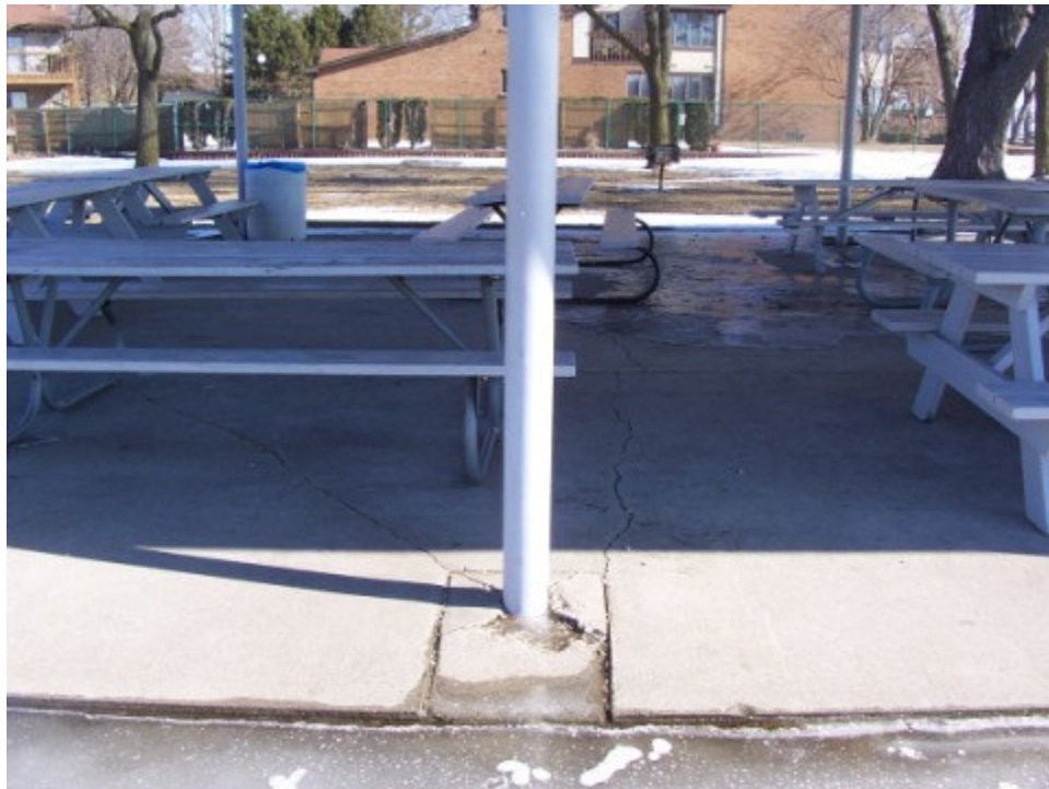
Photograph No. 4: Looking north at post #9. Note settlement and cracking of slab around the pole and cracking of slab within shelter footprint. Also, note standing water around perimeter of slab.
