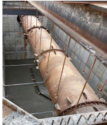
Figure 2 GBC-DVS flume pipe
