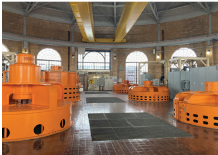
Conner Sewage Pump Station. Courtesy of GLWA
