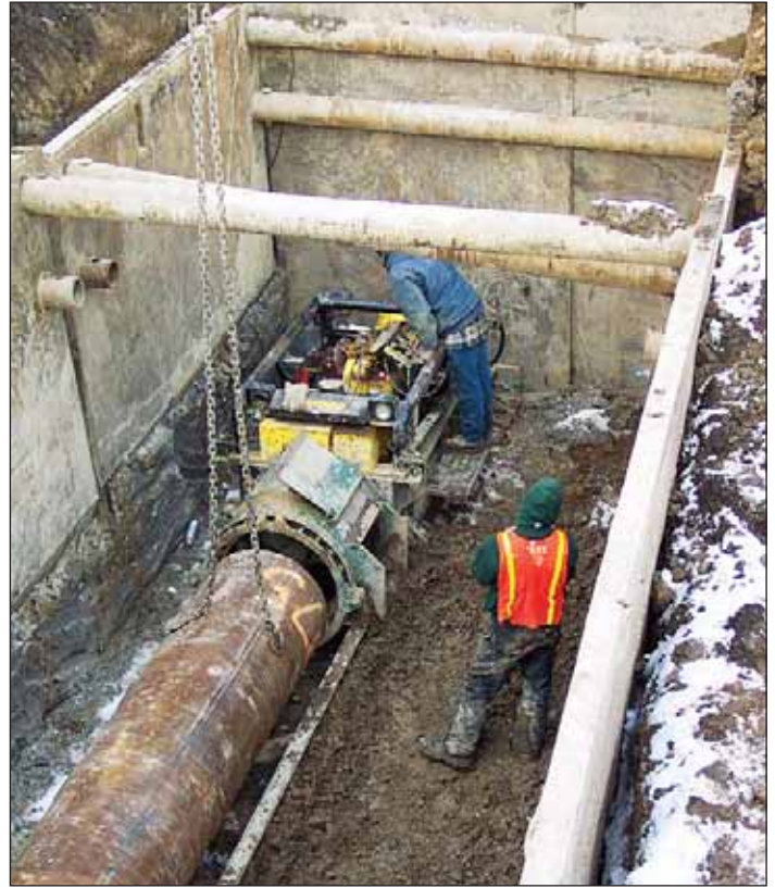
A three-mile force main constructed through urban and environmentally sensitive areas, connects the North Huron Valley/Rouge Valley system to the Downriver system and basin, providing more in-system storage capacity for wet weather flows.
