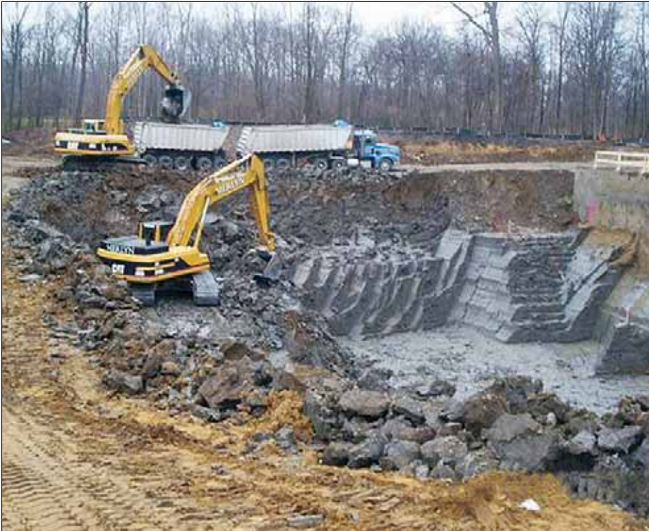
Because of the basin's 50-foot-depth, two excavators worked in tandem to more easily transfer the spoils to the trucks, provided by John D. Osborne Trucking.
