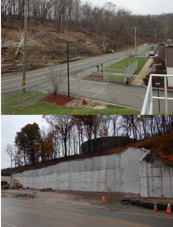
Figure 7: Construction of the pump station required cutting back the hillside and installing a retaining wall.
